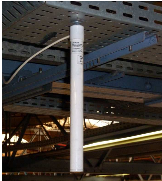
Antenne CISCO AIR-ANT1728
